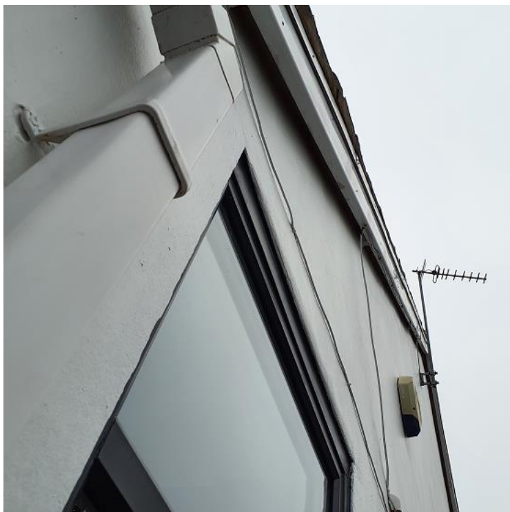
Photo 6. Wide/shallow gap behind barge board on west-facing gable.
