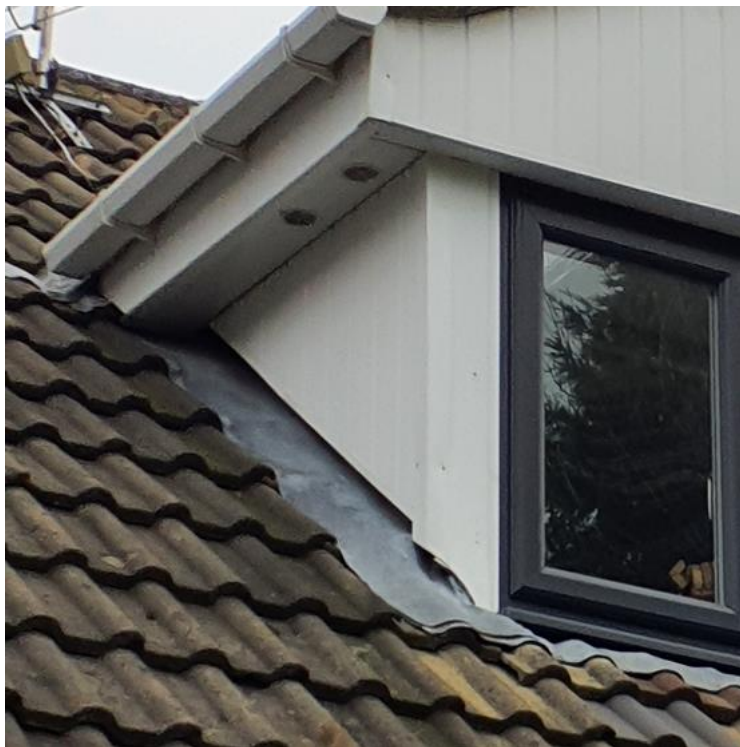
Photo 7. Possible gap behind cladding.
