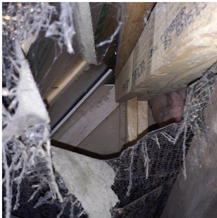
Photo 14. Torn roof lining and light penetration.
