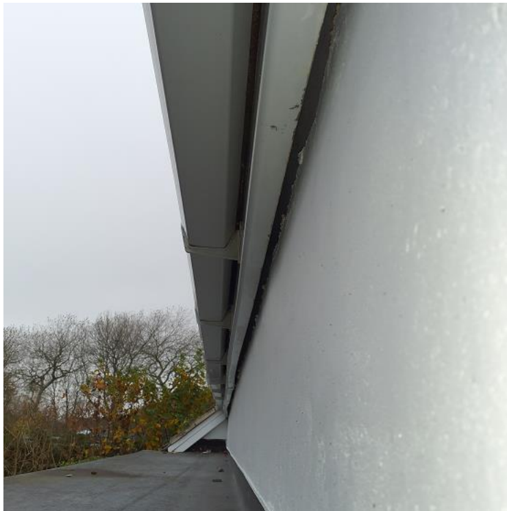
Photo 9. Gap behind fascia above the rear patio door unit.
