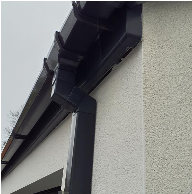
Photo 11. Detached fascia on the garage.
