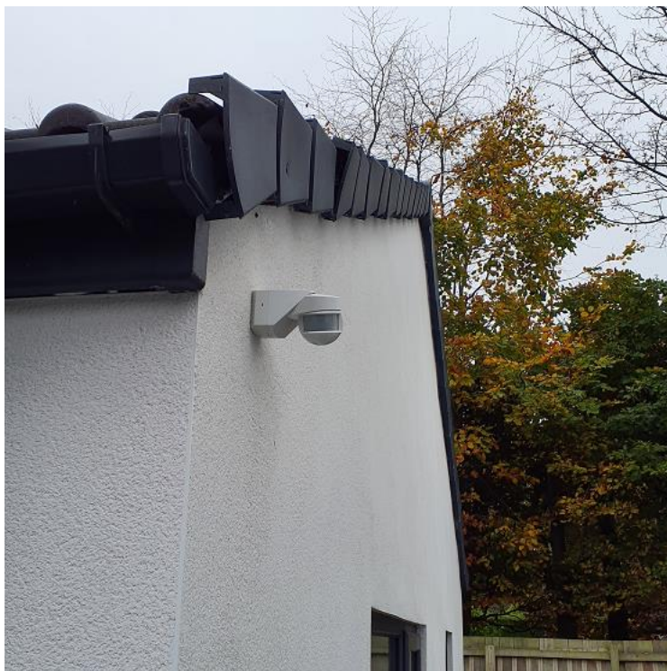
Photo 10. Displaced dry verge units on the garage.
