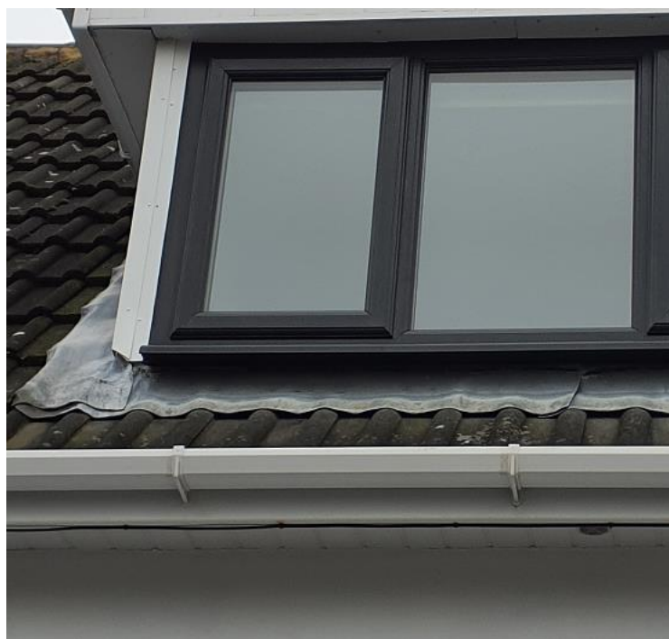
Photo 8. Gaps below lead flashing.
